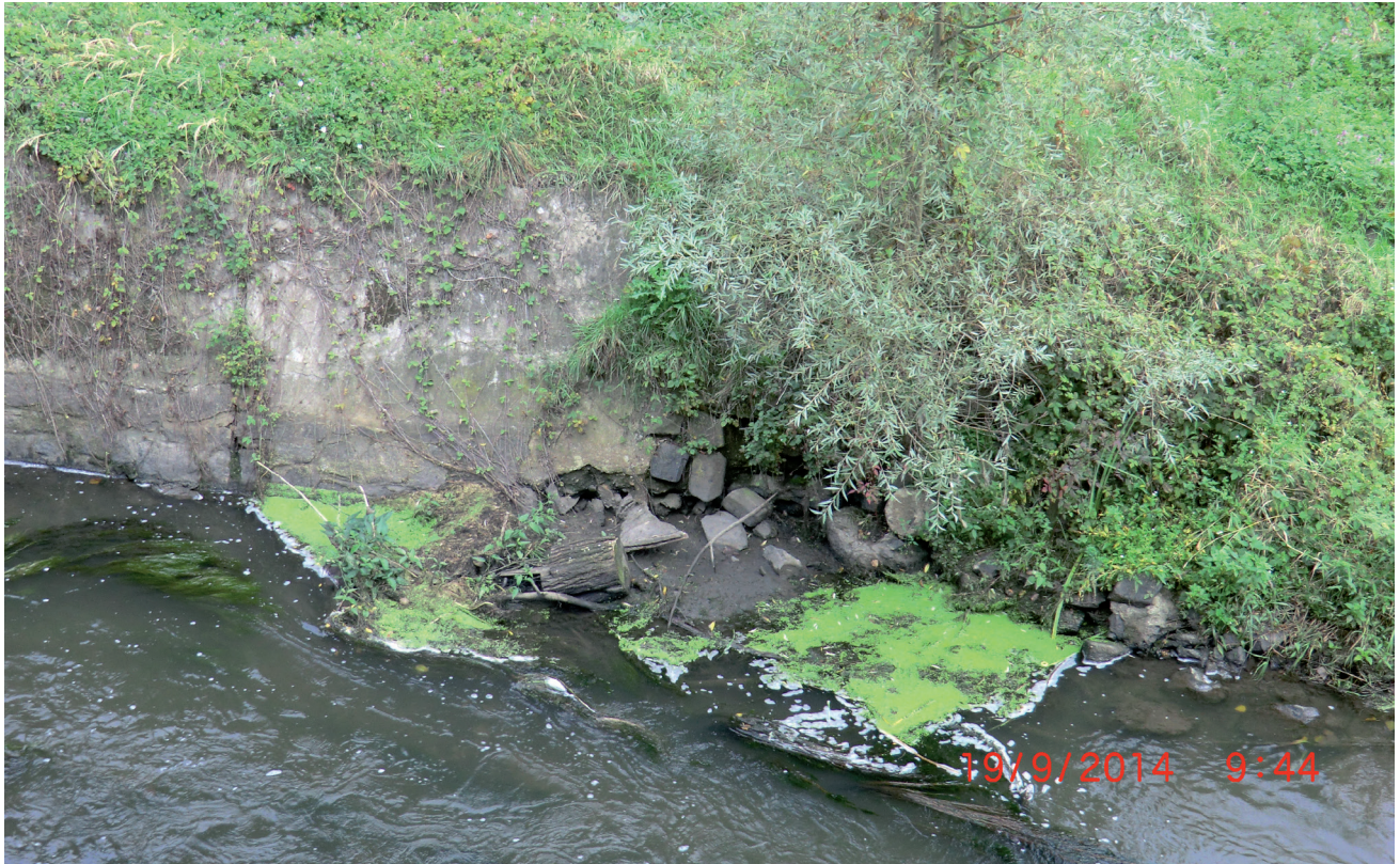
Fig. 10 Destroyed concrete adaptation shore. Reach BIL029, because of the riparian vegetation and water destroying the concrete bank fortifications and lateral water erosion the situation before the bridge over the river could eventually disrupt the bridge structure and scour the adjacent road.
