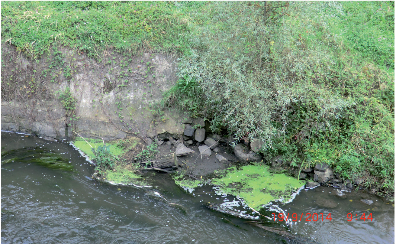
Fig. 10 Destroyed concrete adaptation shore. Reach BIL029, because of the riparian vegetation and water destroying the concrete bank fortifications and lateral water erosion the situation before the bridge over the river could eventually disrupt the bridge structure and scour the adjacent road.
