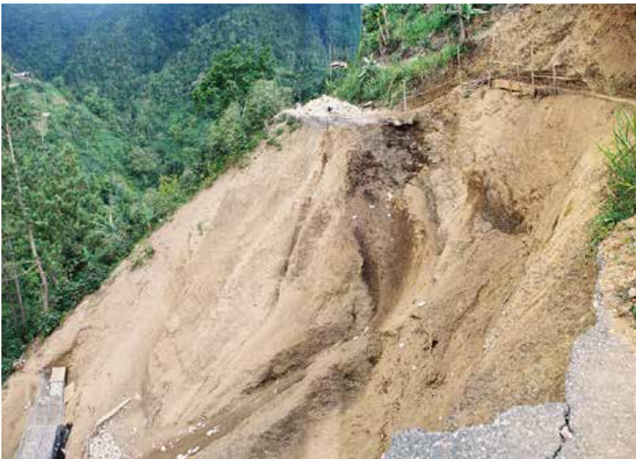
Fig. 3 Landslide on the B1 road at Section in Portland Parish, Jamaica. This event severed much of the local coffee production industry from the ports used to ship the product to market. (The picture is a photo-collage and some distortion is inevitable.)
