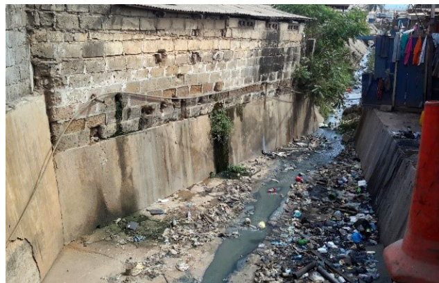
Fig. 3 Pipelines found in drains in La.
