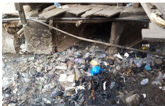
Fig. 2 Pipelines found along and in drains in Chorkor.
