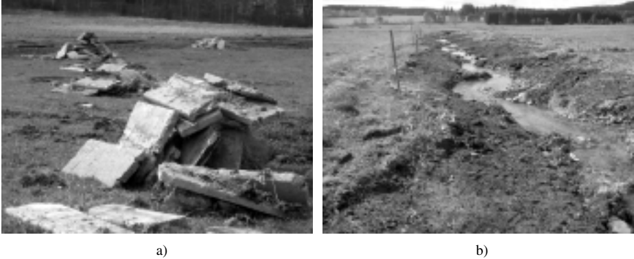
Figure 3: Restored channel of the Sviňovický Brook: a) removed concrete revetment, b) restored channel, closing of the subsurface drainage outlets – situation spring 2005. Photo: Matoušková
